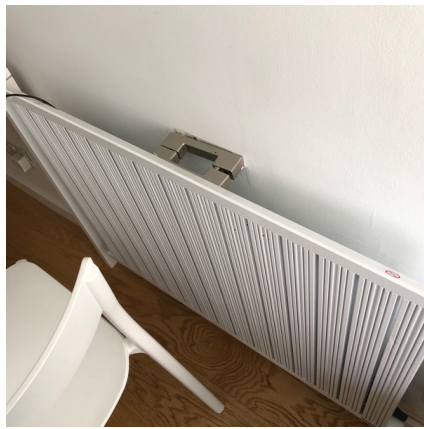
Loose radiator to kitchen that needs securing.
